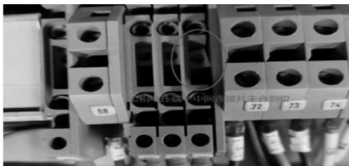
图2 相电压端子中间连接片未合到位 Fig. 2 The middle connecting piece of terminal of phase voltage is not closed to final position
